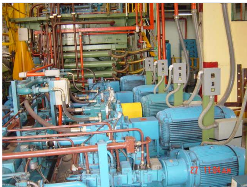
Figure C-1: Upgraded hydraulic system, on floor at rear of press.
