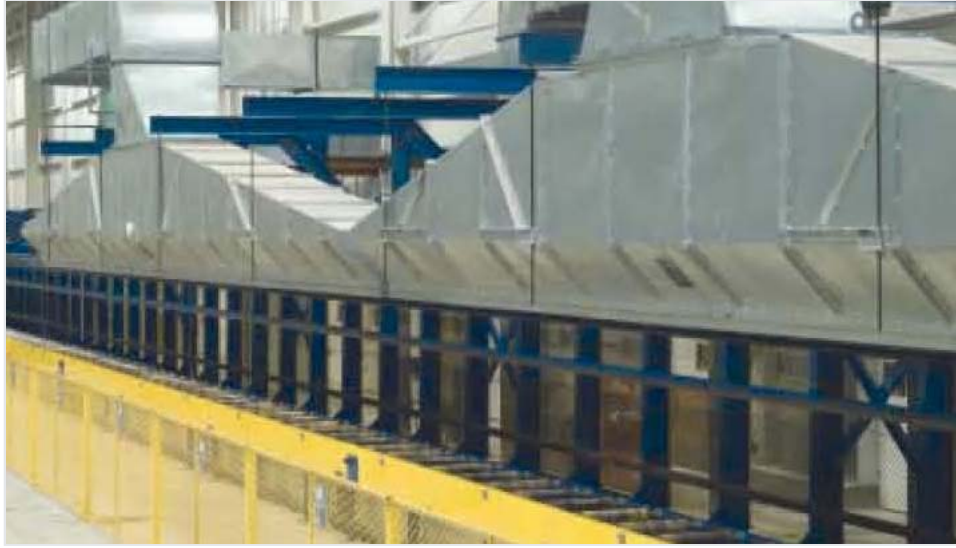
Figure C-17: Air cooling duct located over run-out (Photo courtesy of Granco Clark)
