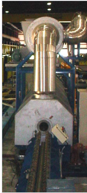
Figure C-12: Log furnace with waste heat recuperator (Photo courtesy of OMAV)
