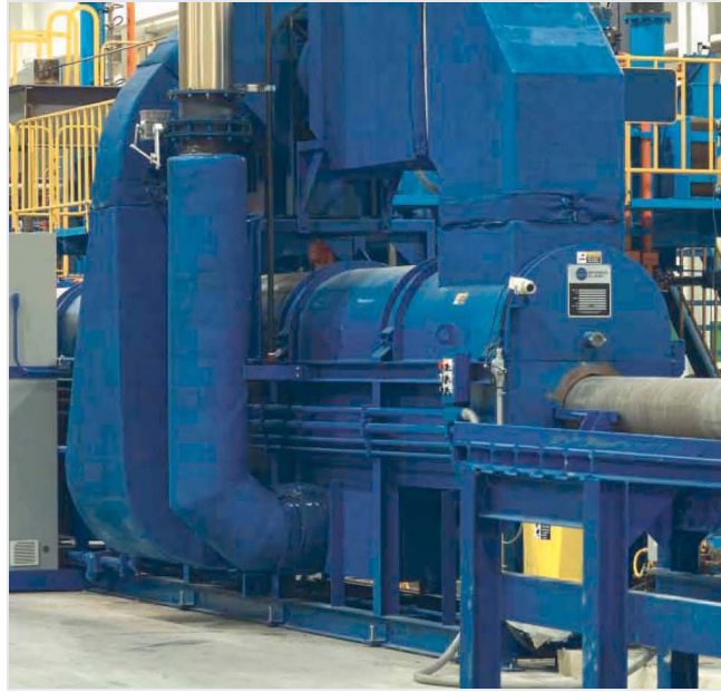
Figure C-13: Log furnace with hot gas recirculation (Photo courtesy of Granco Clark)
