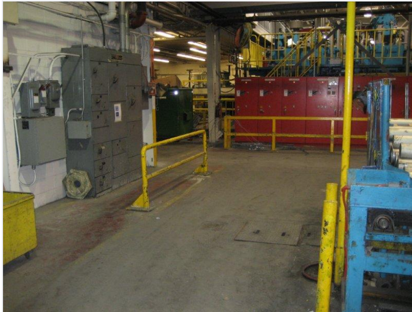
Protected Switchgear with Guard Rail
