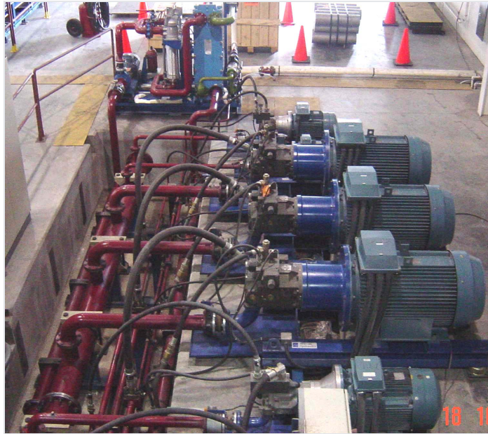
Figure 5-5: Floor-mounted pump layout with three main pumps, three auxiliaries, one spare, “kidney loop” filtration, and plate-type heat exchanger at rear (Photo courtesy of Presezzi Extrusion)
