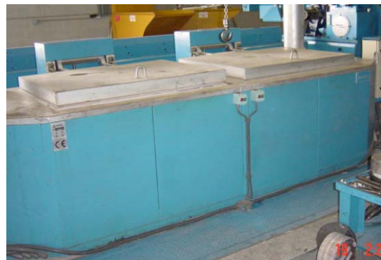
Figure 10-1: Box-type die heaters (Photo courtesy of Gia)
